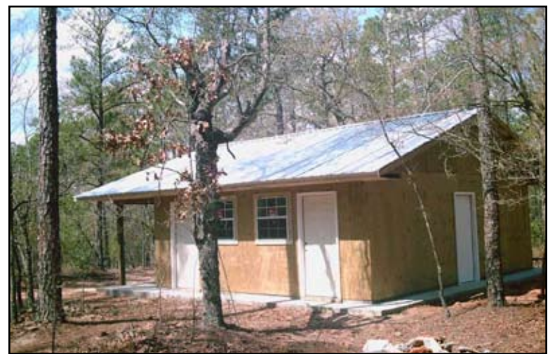
The construction of this shower house at the Maubila Scout Reservation in Jackson, Alabama was partially funded by the SR-1B grant
