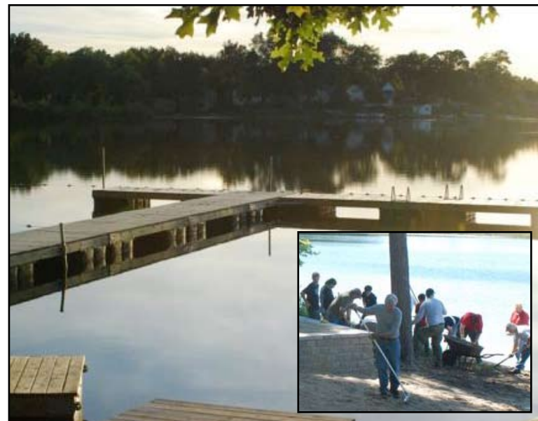
Chippewa Lodge received a matching OA Service Grant to help construct swimming docks and a waterfront retaining wall.
